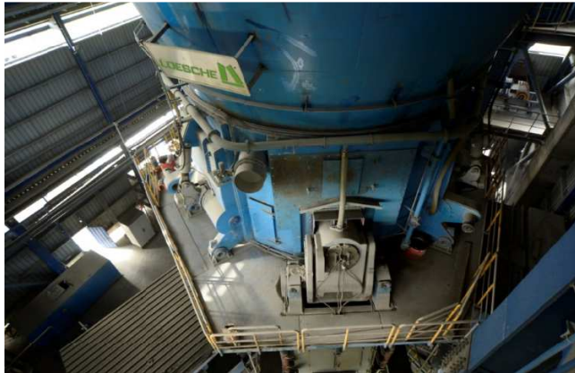
The LOESCHE cement mill in operation in the cement plant Banyuwangi, Indonesia
